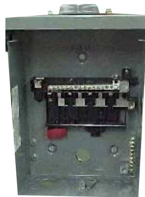
Figure 4-7; BBX 100A (BBX-F18) Square-D, 8-position For multiple power supply applications.
